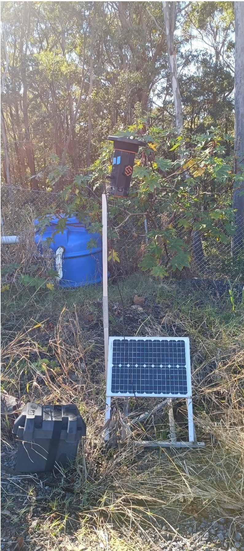
Photograph 10 – Real time monitor installation
